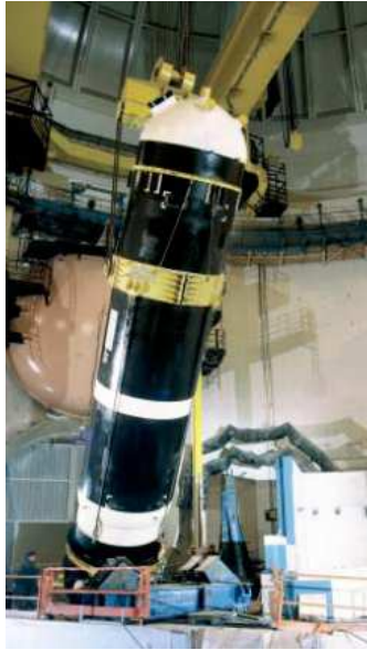
Figure 3.16 - Erection of a Pressuriser in a reactor building. (Courtesy of Areva NP: http://www.aveva-np.com/ ).
