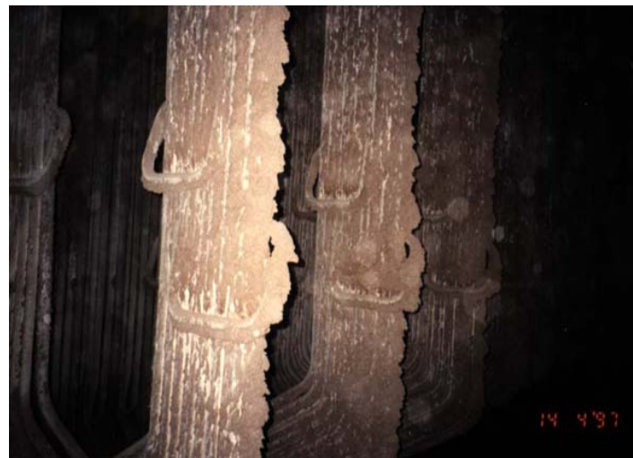
Fouling of a superheater in a biomass boiler
